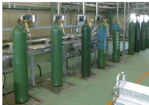
Gas reclamation and filling facilities
